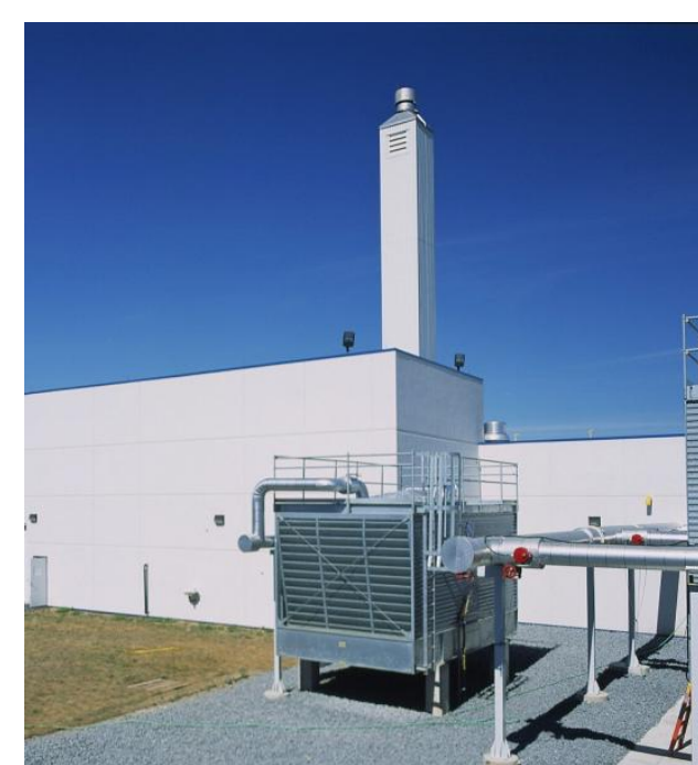
Figure 5 Markham District Energy plant. (Source: Town of Markham)
